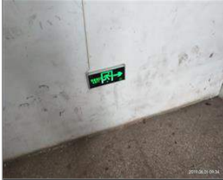
Photo of fire safety equipment Evacuation indication sign.jpg
