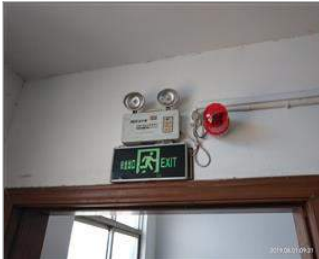
Photo of fire safety equipment Exit sign emergency light and fire alarm.jpg
