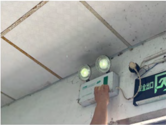
Fire facility onsite testing
