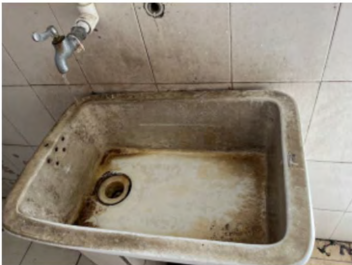
NC Missing toilet paper and soap
