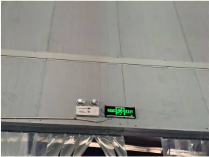
Exit sign and emergency light
