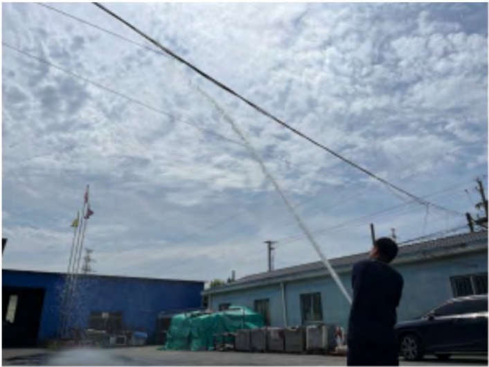
Fire facility onsite testing
